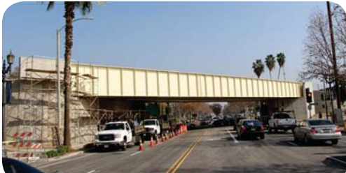
The final bridge of the 24 bridge structures completed on the project spans the intersection of Huntington Drive and Second Avenue in the City of Arcadia.
