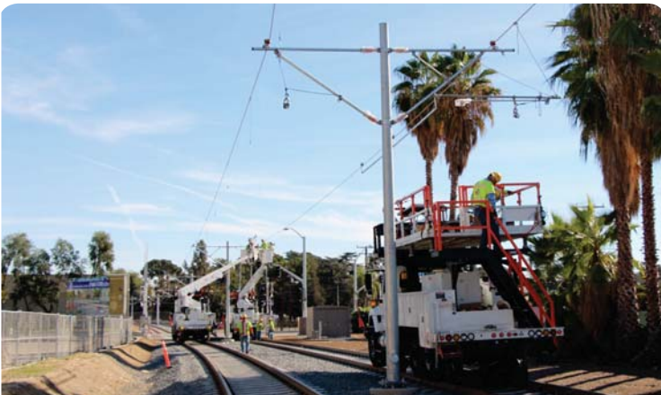
Seen here in Monrovia, many different pieces of specialized on-track equipment are utilized to install the Overhead Catenary System.
