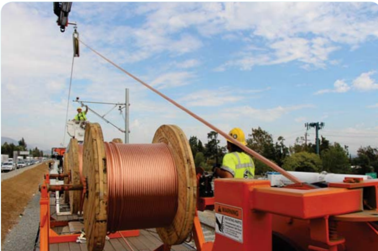
Workers in the 210 Fwy median through Arcadia are using a track mounted boom truck and bucket truck to thread the "messenger wire" from large cable reels as part of the Overhead Catenary System (OCS).
